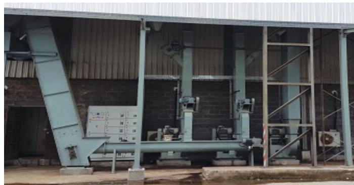
Figure 3. Pre-cleaning system installed at the kernel crushing plant.
